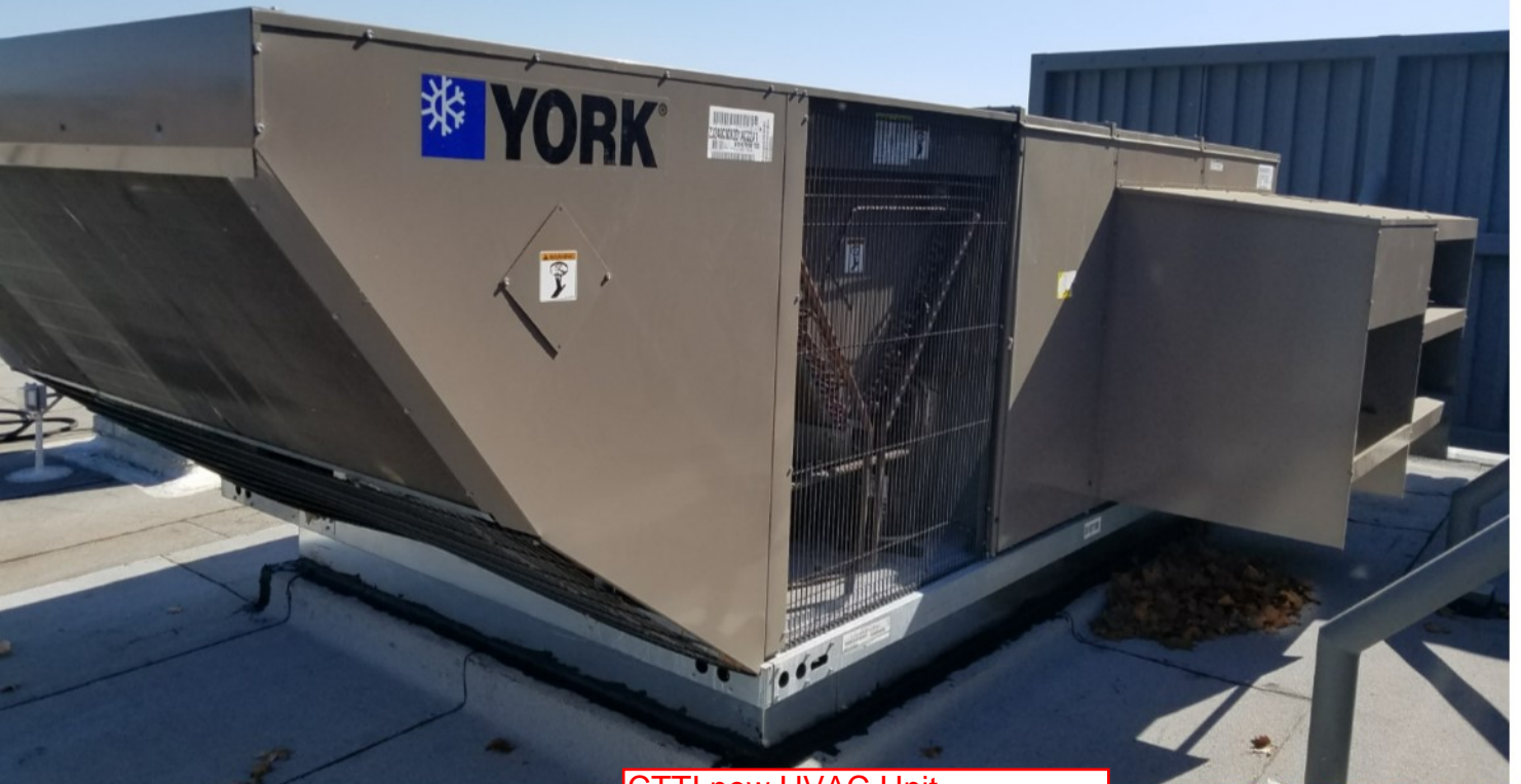
CTTI new HVAC Unit
