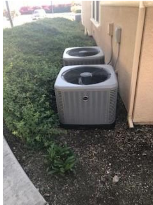
New Phase II condenser
