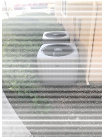
New Phase II condenser
